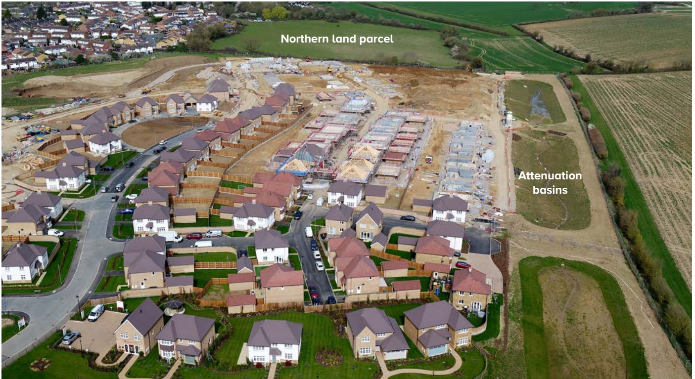
Aerial view of Redrow's site, showing new properties which front onto Western Road in the foreground. The northern land parcel, which will accommodate 126 new homes, is labelled in the background.
